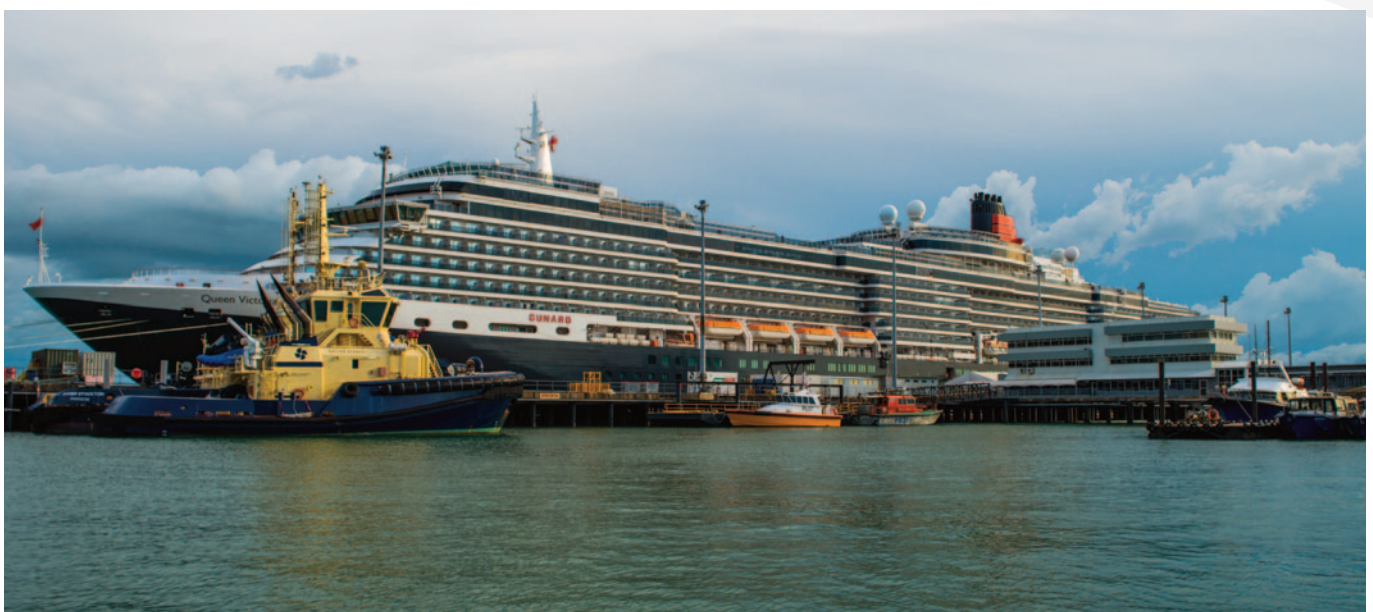
Work is progressing to accommodate future larger cruise ships at Fort Hill Wharf
